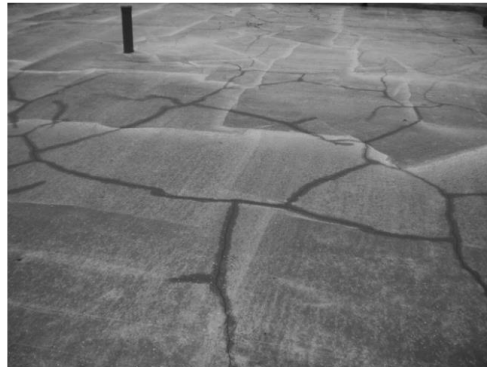
Figure 1: Early-age cracks in concrete slab (from [1]). Space between cracks is around 1m.
