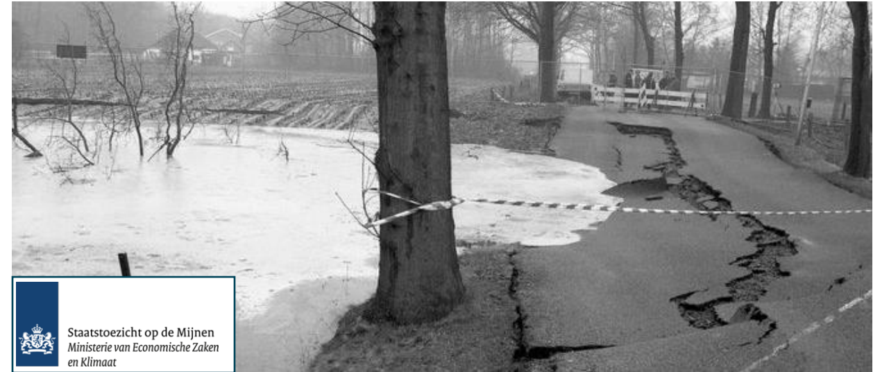
Sinkhole Hengelo/NL 1991: diameter 30m, 4.5m deep
