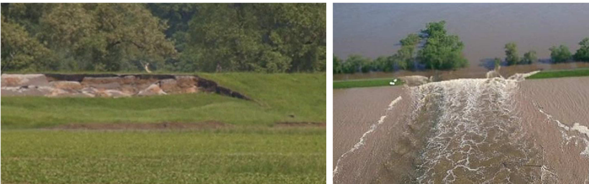
Levee Failure (Breitenhagen, Germany, June 2013). Left: initial stage of the failure process, probable cause was instability. Right: breach in progress.
